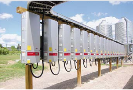
/ 200 kW system, Canada
