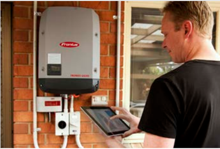
/ 3 kW residential installation, VIC
