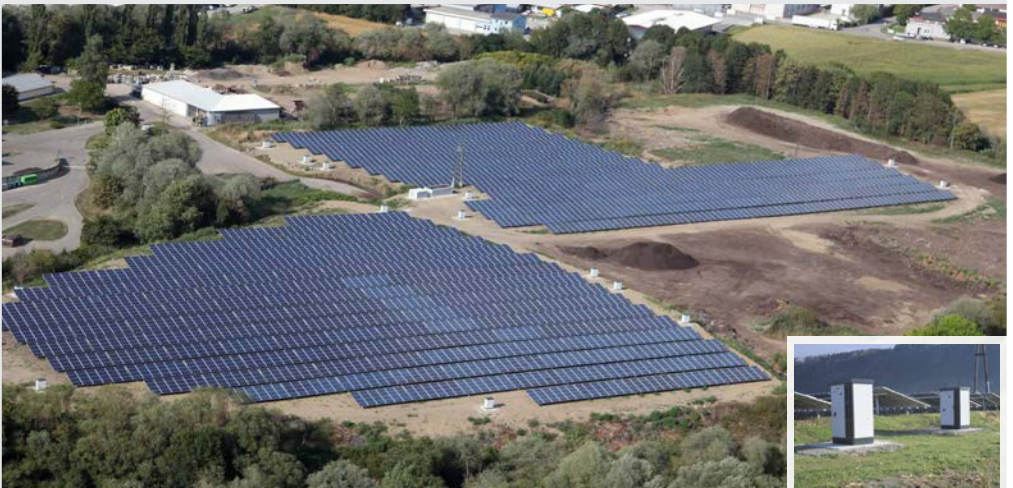
/ 1.5 MW plant, Austria
